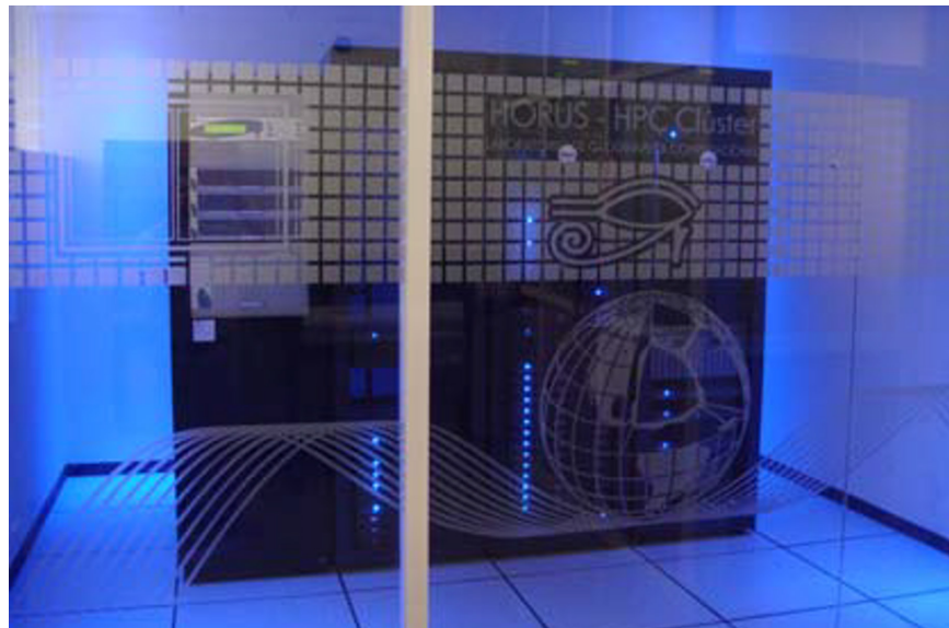
Figure 6. HPCC – Horus at the Geosciences Center – UNAM. Some of its main characteristics were (as per 2010): 188 computing cores (AMD-based), 500 GB of RAM, 2×15 TB RAID 5 storage DAS (Direct Attached Storage), Primary (30 kVA) and secondary (2 kVA) UPS units, and a redundant cooling system.
